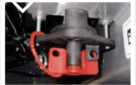
LOG- OUT TAG- OUT BATTERY MASTER SWITCH
