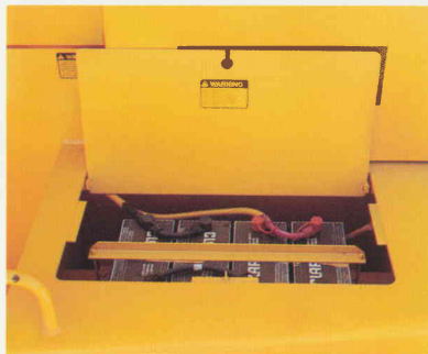
Battery box positioned for convenient inspection.
